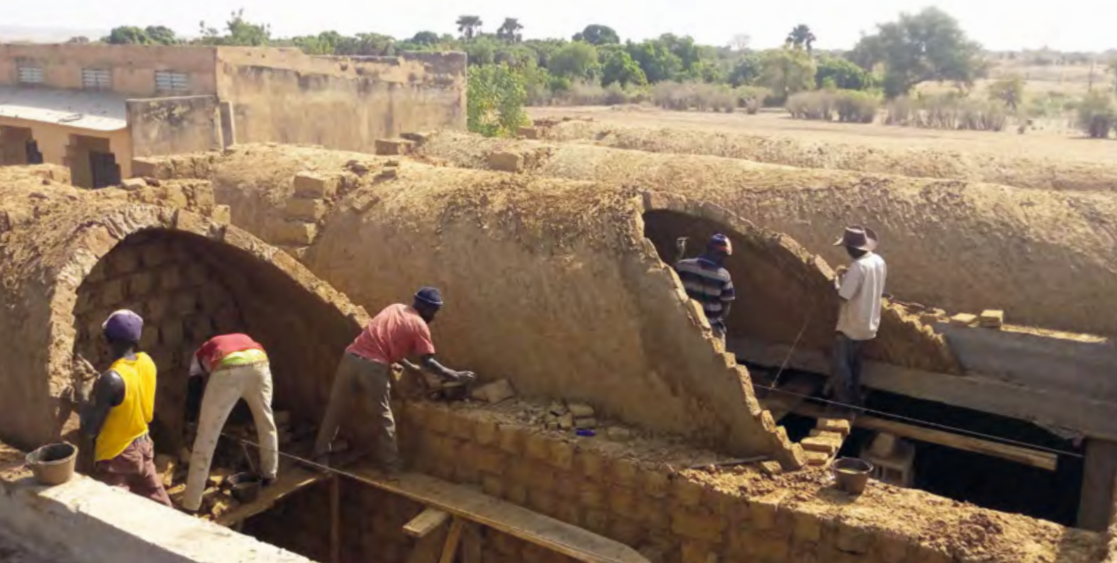
The college of Lontou (Kounda78) construction site (top) and finished building (bottom).
